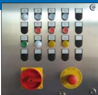
Bedienfeld / Operation panel
